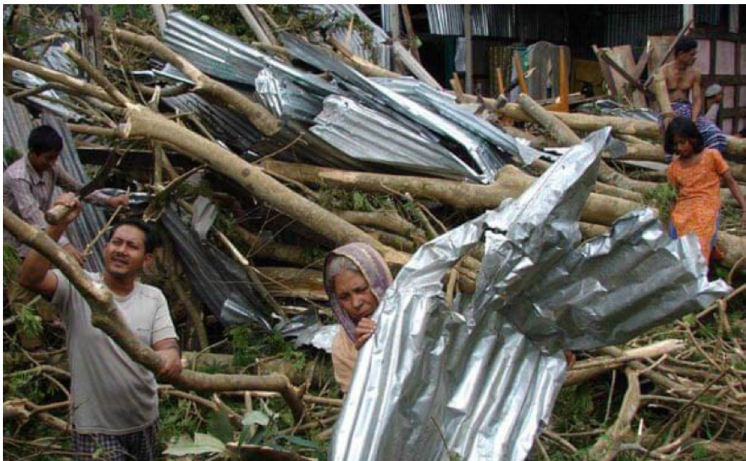
Residents of Char Bangla sift through their damaged houses for usable material in the aftermath of Cyclone Aila. Photo by The Guardian.
