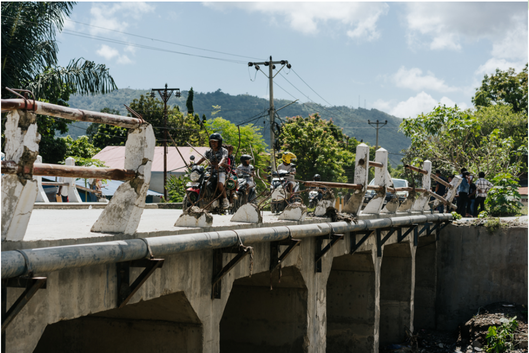
Damage caused by floods in Dili, Timor Leste. Photo: Oxfam in Timor Leste
