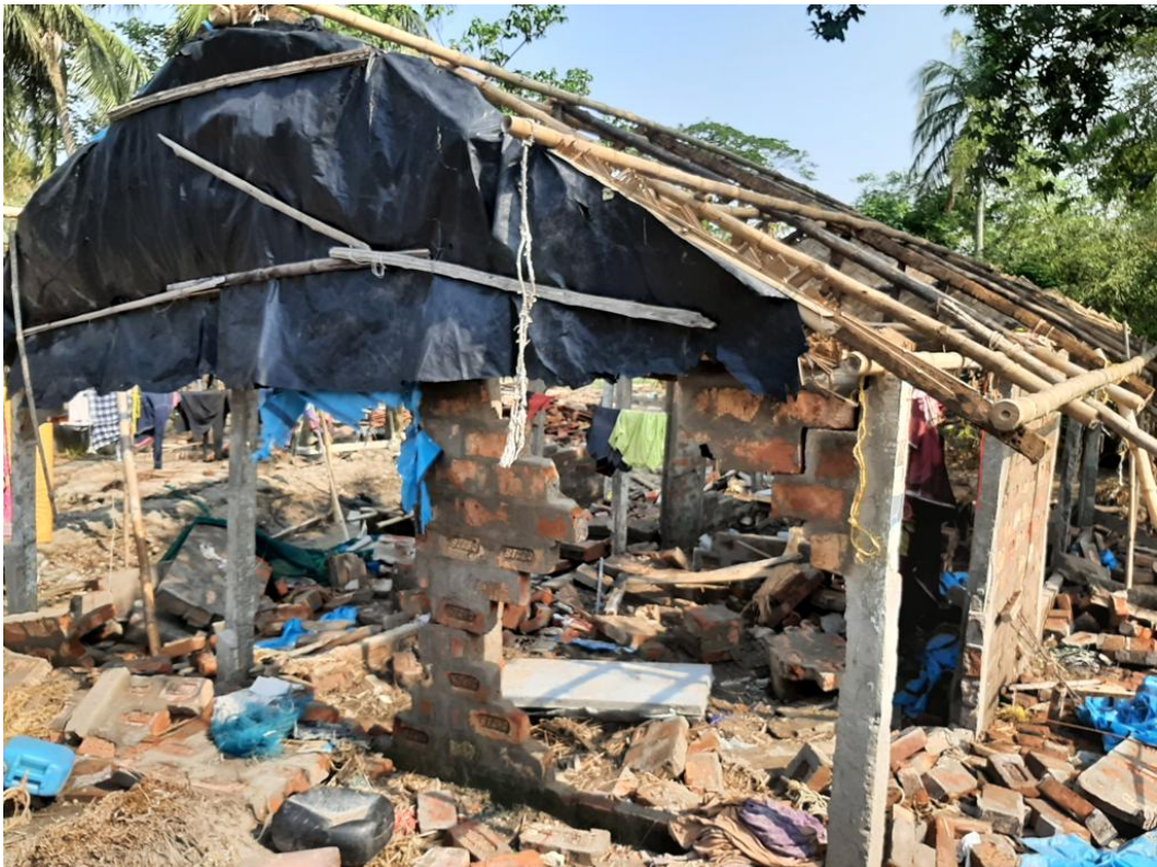
House heavily damaged by Cyclone Yaas. Pinaki Halder / Landesa. June 2021
